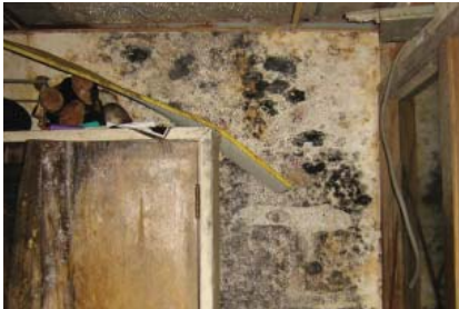
Moisture Problems & Building Impact
