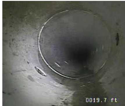
Sigma's sewer camera
